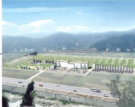
HVDC Converter Station 1000 - 12000 MW, Classic
